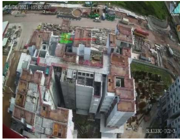
2. Worker under lifting load
